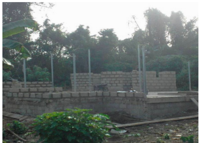
On-going construction of the gari and cassava dough processing facility at Amanase Aboabo, at Ayensuano District Assembly
